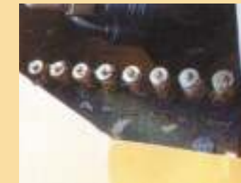
The central measuring point in the engine compartment makes it possible to check all relevant working pressures at any time within some seconds. Your advantage: immediate diagnosis = cost saving.
